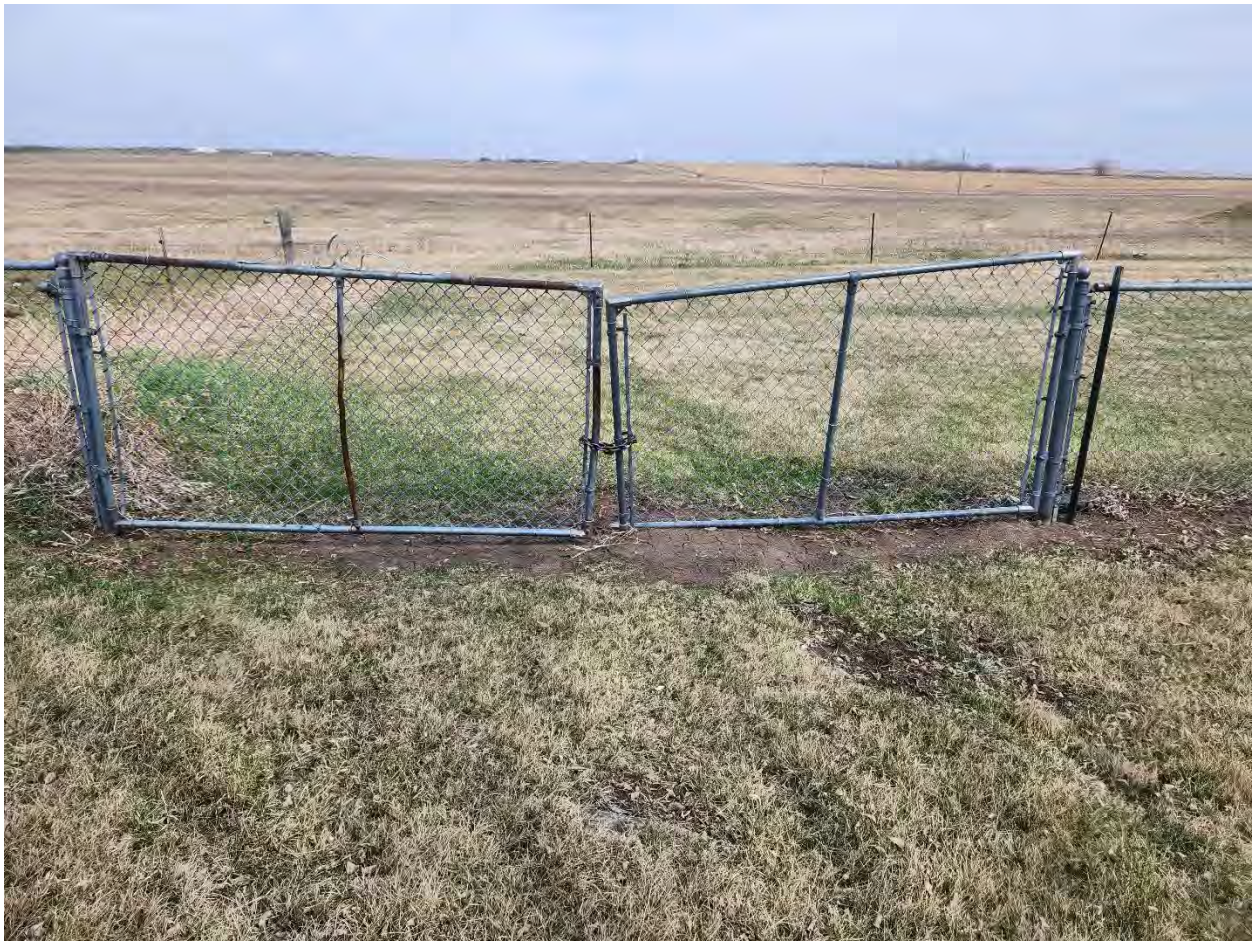
Repair or replace (broken on the bottom)
