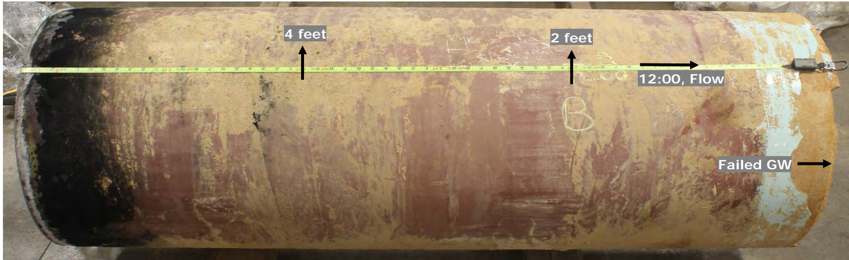
Figure 7. Photograph of PS B after removal of the protective wrappings. The tape measure indicates the distance from the D/S end of PS B.
