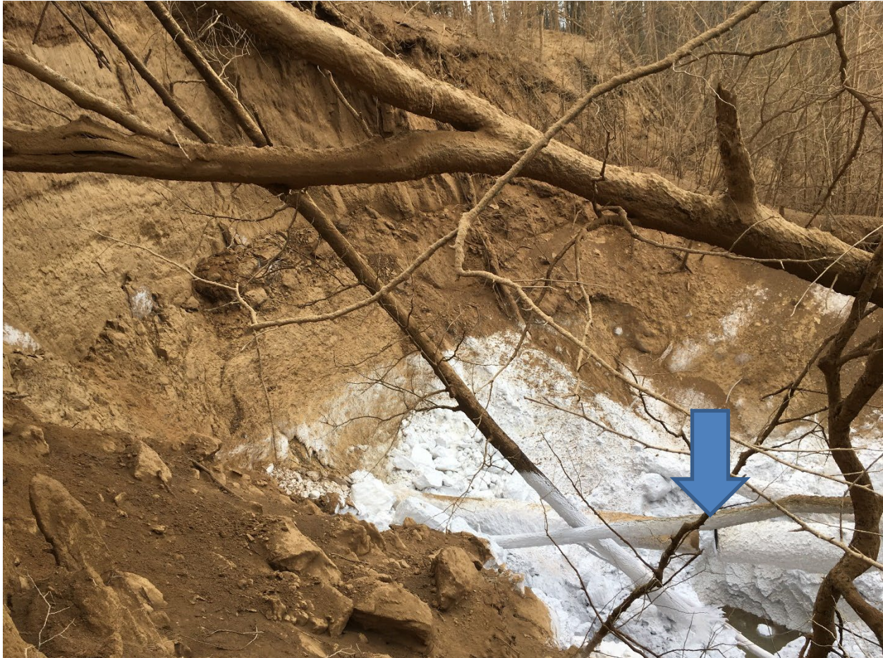
Figure 3: Crater Created by the Rupture Containing Fallen Debris (dry ice, and the failed pipe sections) (Blue Arrow is Pointing at the Pipeline Separation)
