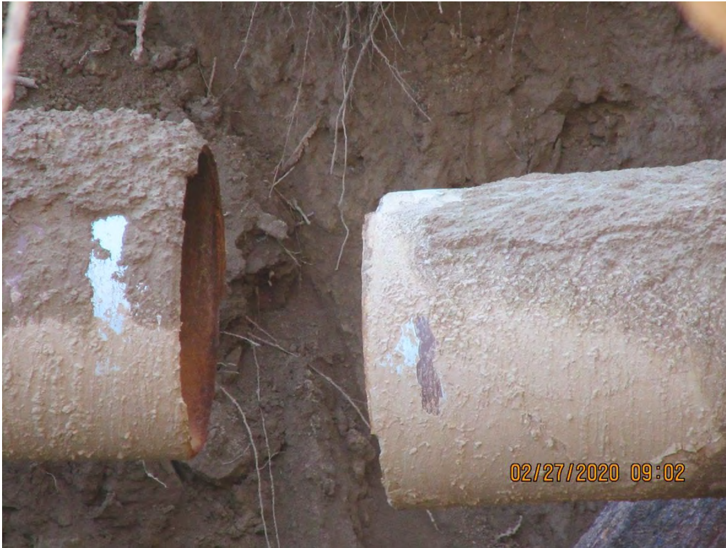
Figure 8. Delhi 24-inch Transmission Line Failure - As-Found Condition at Girth Weld
