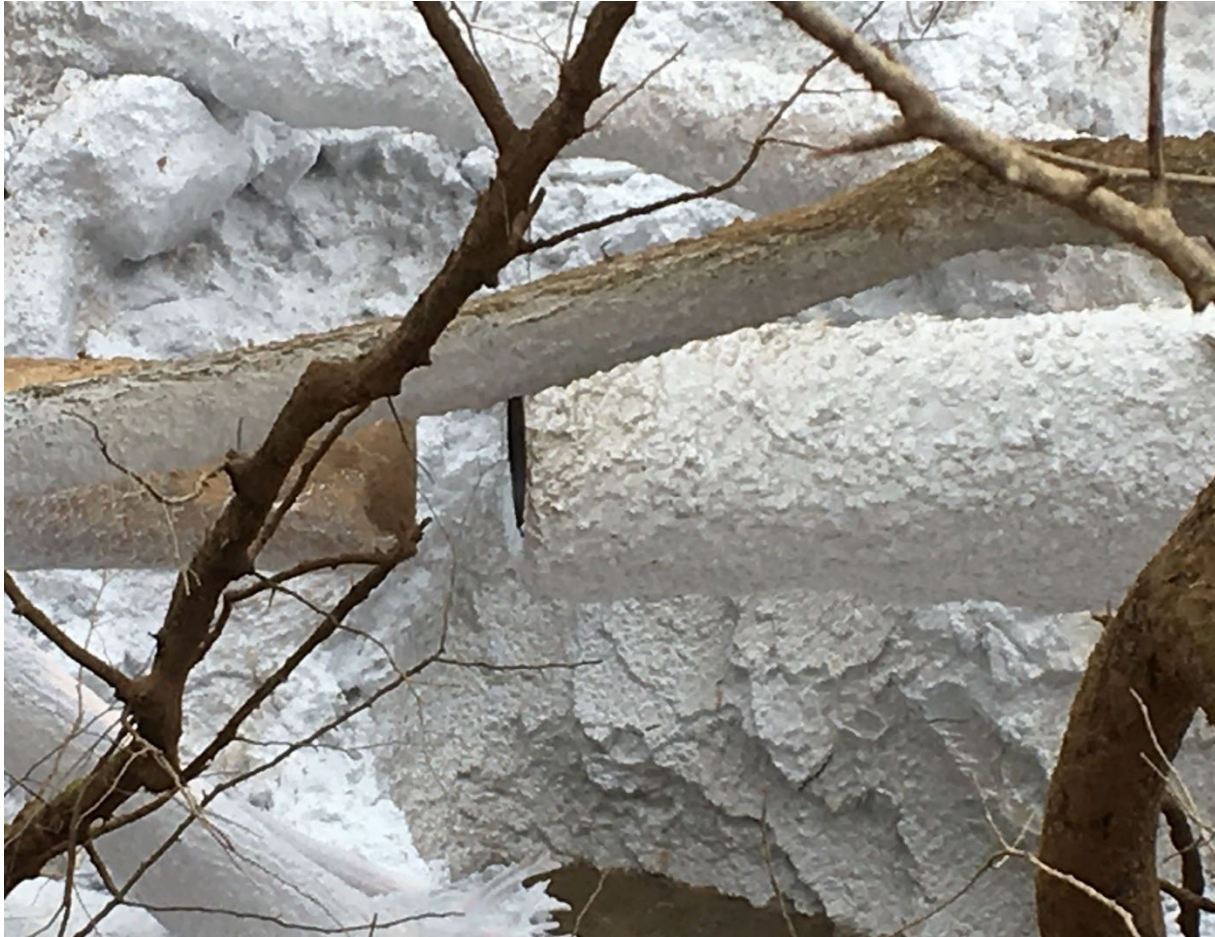
Figure 4: The failed pipe sections shown separated by a few inches.
