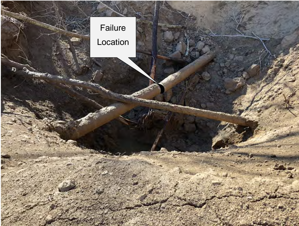
Figure 7. Failure Location (Upstream to Downstream)
