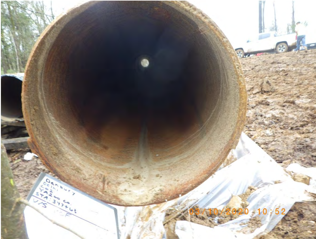
Figure 11. Internal Condition of Pipe Sample During Removal
