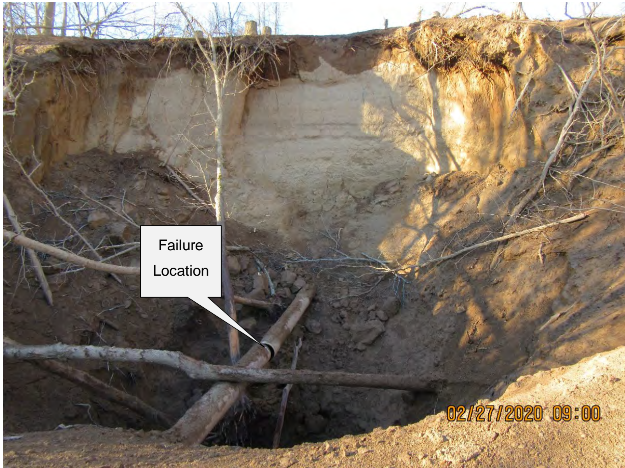
Figure 6. Failure Location (Upstream to Downstream)
