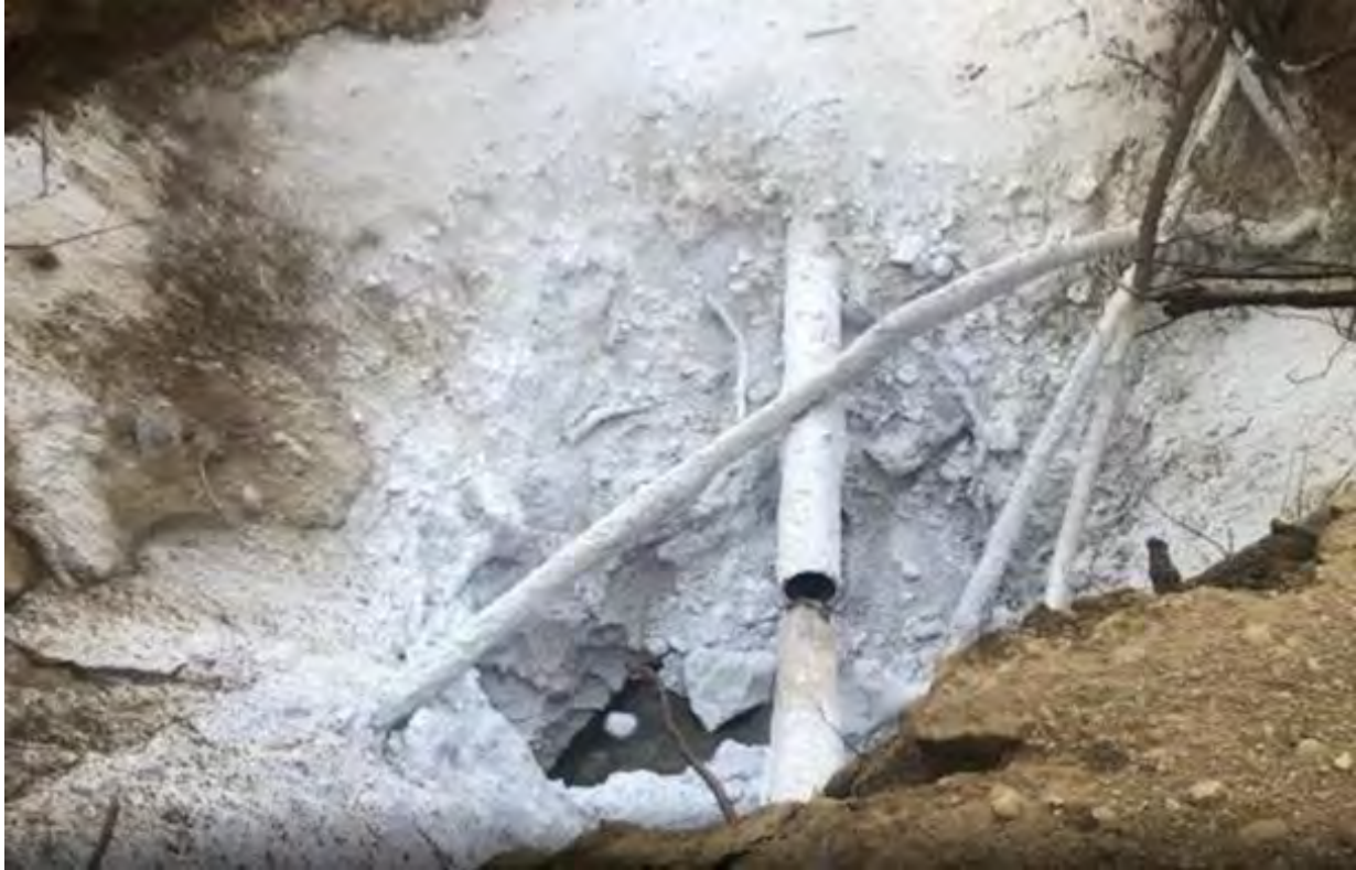
Figure 4. Post-Incident Photo of Failure Location (Downstream to Upstream)
